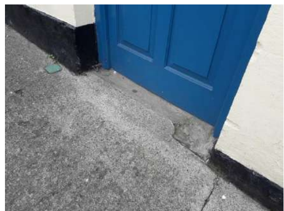
Fig 46 – issue with water runoff at threshold
