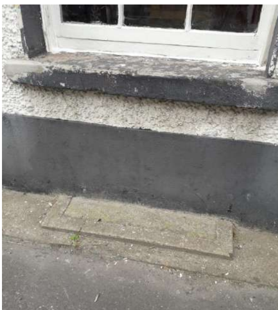
Fig 42 – blocked opening to basement
